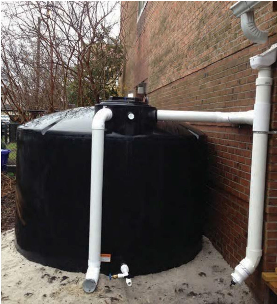
Figure 4.23. Example cistern application (photo: Marty Morganello).
